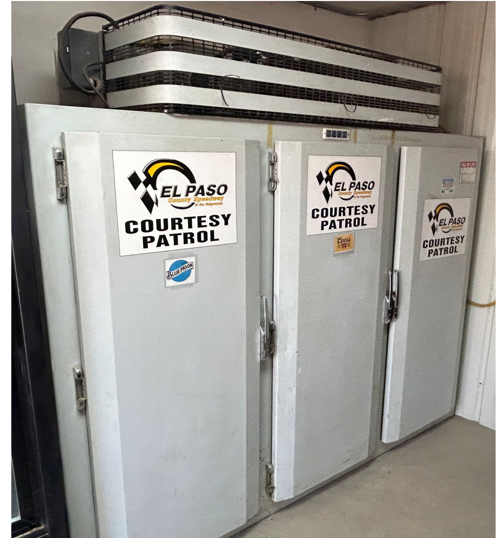
Beer Dock Refrigerators
