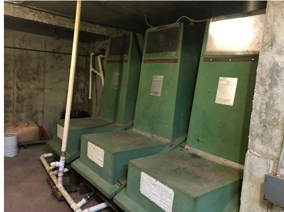
Composting units in vault, to be removed
