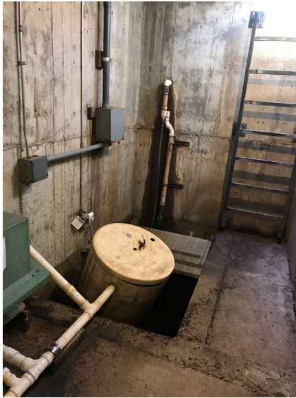
Filter tank in vault
