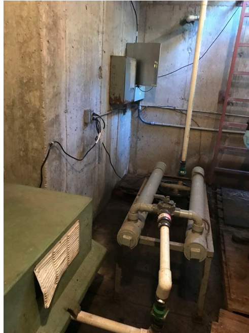
Vault equipment to be removed
