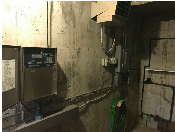
Irrigation controls in vault
