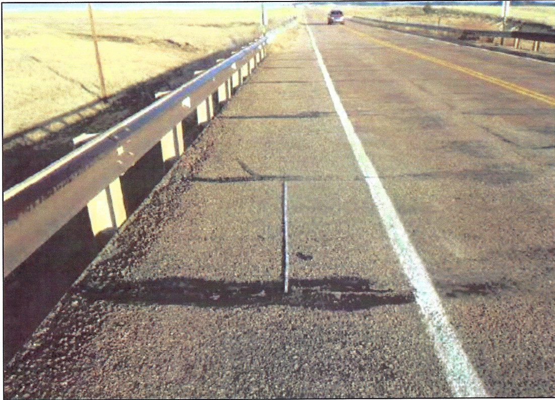
Figure 2. Structure EPC009104.37A existing bridge deck condition. (Engineering Operations, 2018)
