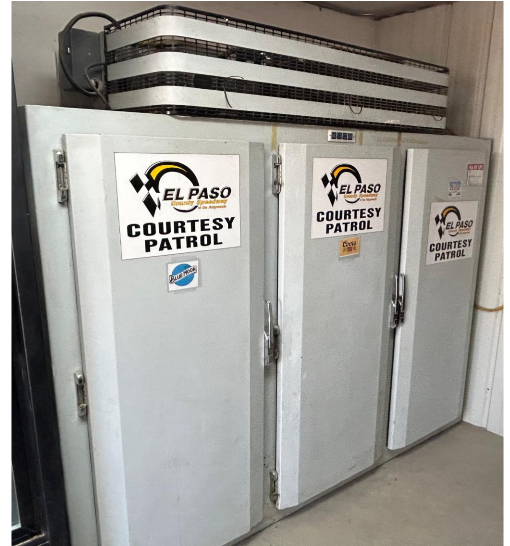
Beer Dock Refrigerators
