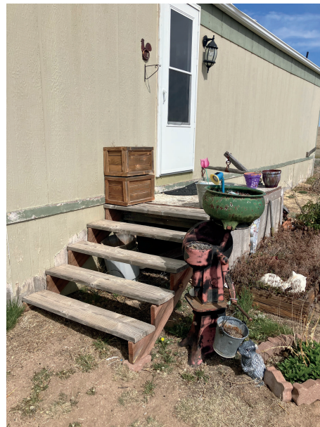
BEFORE: Unsafe Exterior Access
