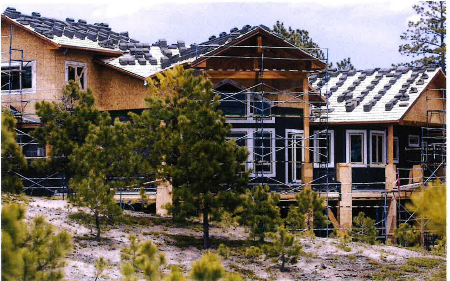
A home under construction in the Cathedral Pines development in Black Forest is shown in May 2007. the Gazette file
